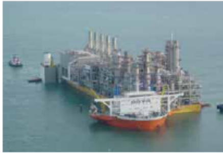
Figure 4. Statoil's Snorvit LNG process barge. Petrotec undertaken mechanical completion of 36 000 t topside.
