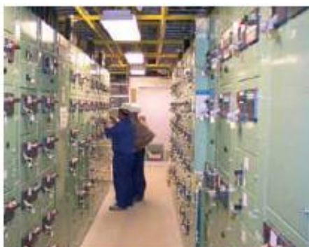
Figure 1. Commissioning of process units, Gulf of Mexico.
